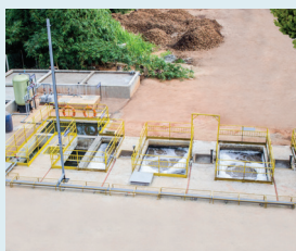
Water and Wastewater Purification
